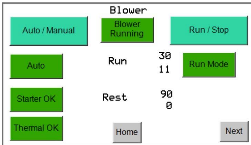
Figure 13. Blower Operation Screen Auto Mode
